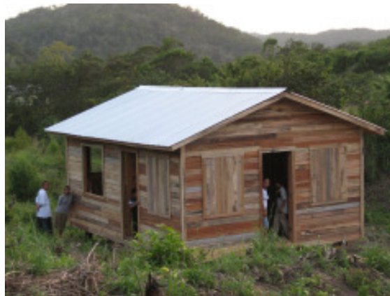
After: The new one-room house the mission team built in San Antonio, Belize for the Romas children.
